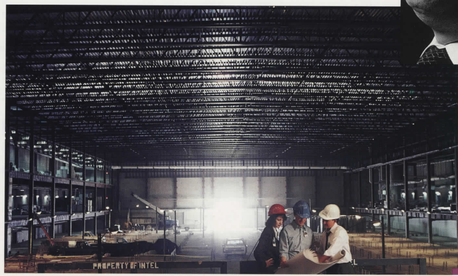
Fab 9, now close to completion in Rio Rancho, New Mexico, is an excellent example of the Administration Group's diversity. Various elements of the Group financed the plant, built it, staffed it, purchased the equipment, and provided security, communications and legal support.
